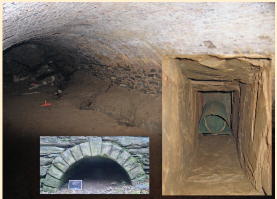
A view of Tunnel A of Tailrace 2. Inset Left: The entry point to the raceway today. Inset Right: A copper drain that was once connected to the Polishing Shop.
